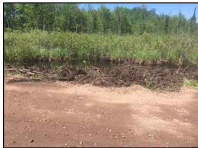
Beaver Dam north of Strand Road culvert #9
